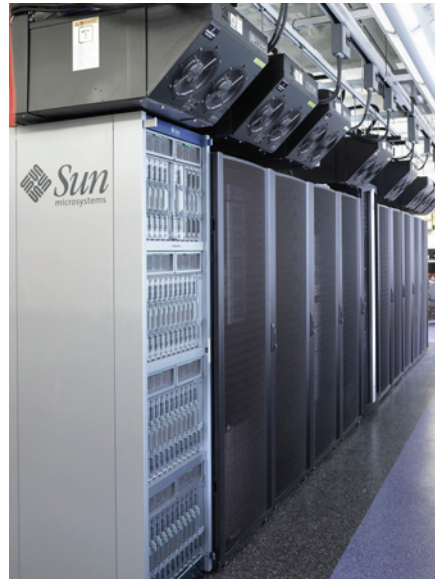
Figure 6. Overhead cooling units can effectively cool high-density racks in raised-floor or slab configurations.
