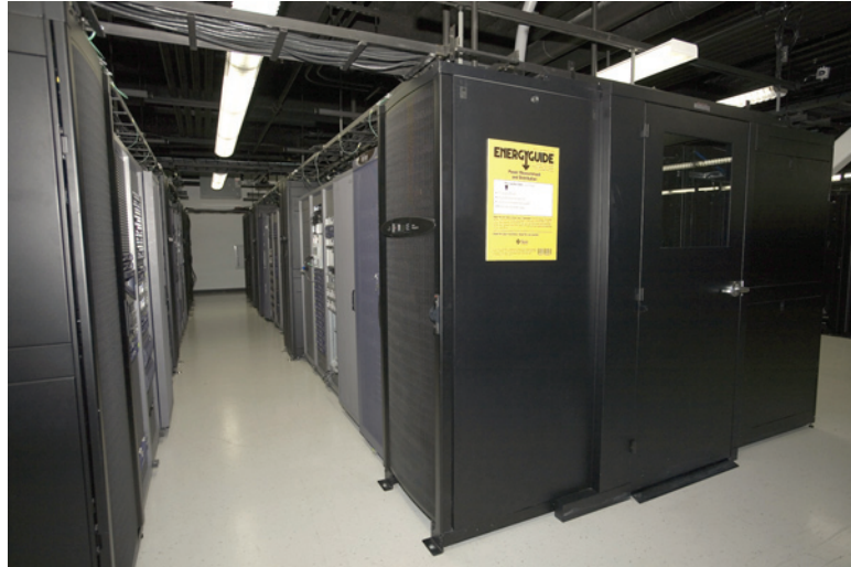
Figure 5. The use of hot-aisle containment with in-row cooling makes pods self-sufficient from a cooling perspective.
